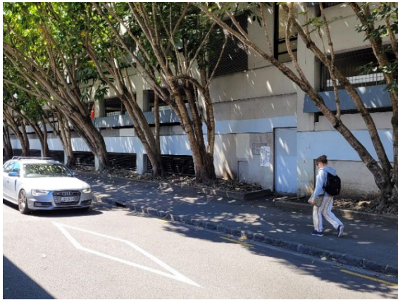
Figure 4.8 Typical presentation of the edge of the existing DTC building to Lower Hobson Street. A closed and inactive façade with trees at the street edge warped by proximity to the existing building.
